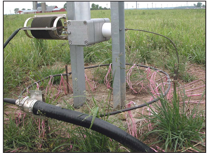
Fig 11-87—Base of one of the elements of the K9DX 9-Circle. Note the high-Q loading coil and the ring (1-meter diameter) made of 10 mm copper, to which all of the 120 quarter-wave radials are connected. K9DX uses 1 \frac{1}{8} -inch coax for the 3 \lambda /4 feed lines.
