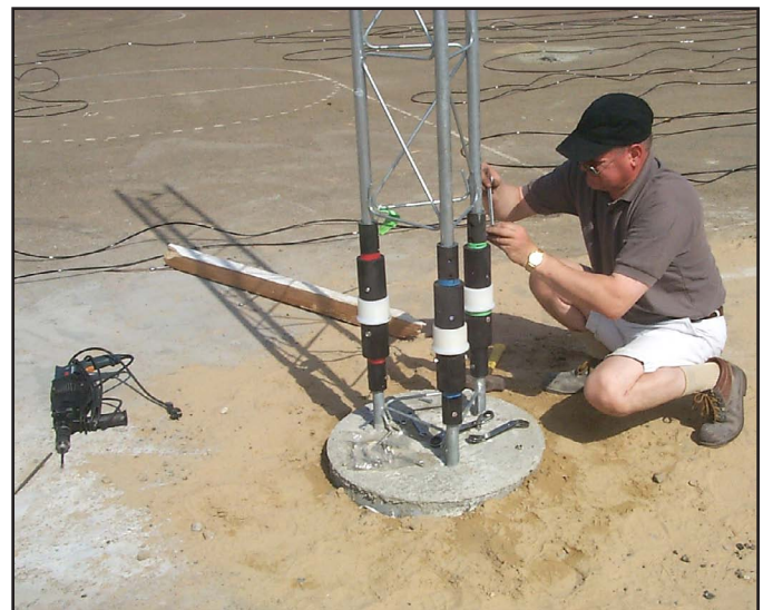
Fig 11-98—Roger Vermet, ON6WU, installing the base insulator on the Rohn 25 tower sections used for the 160-meter Four-Square at A61AJ in Dubai.
